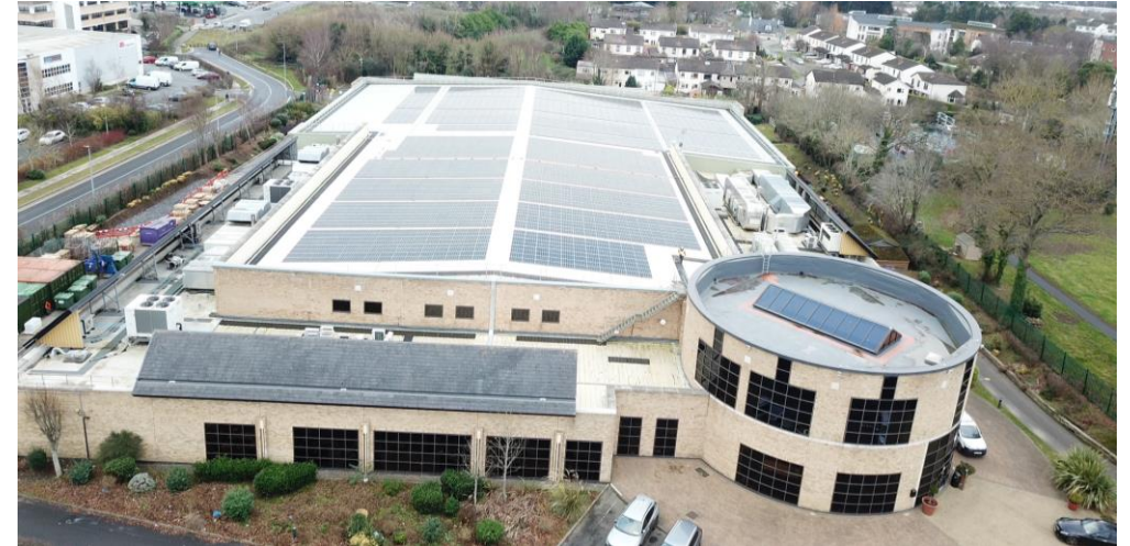
Solar panels mounted on the Renishaw site in Pune, India (top) and work in-progress on solar panel installation at the Renishaw Ireland site in Dublin
